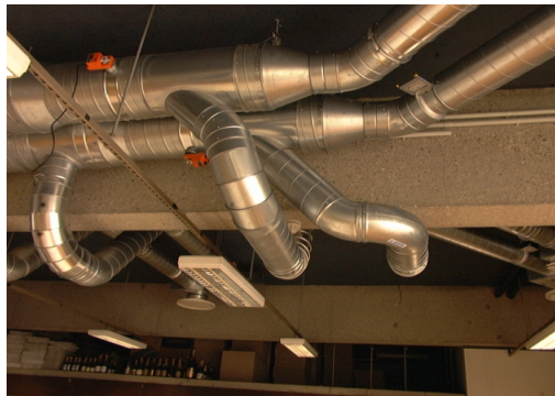
Figure 17 : Views of the duct network of the large hall
