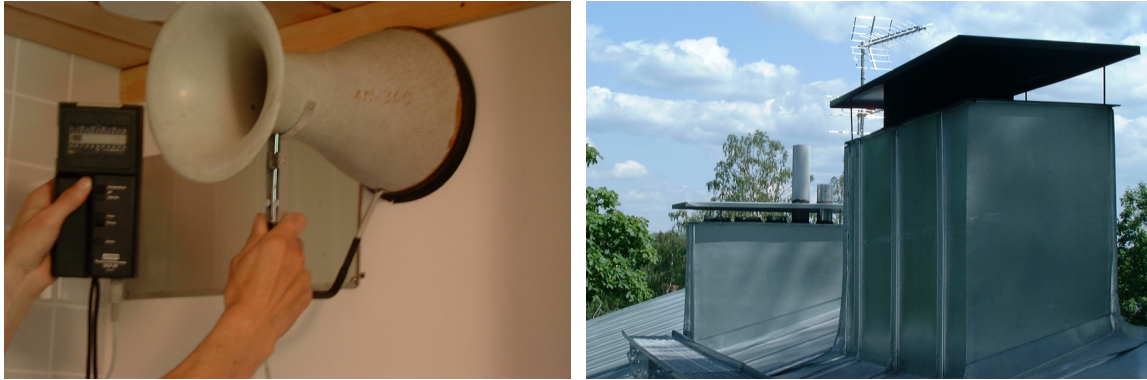
Figure 5. Measuring the airflow rate through one of the exhaust vents. In total there are 8 exhaust vents, of which 4 are fan assisted (bathrooms, sauna and range hood). Each exhaust vent is ducted separately to the roof to reduce cross contamination.
