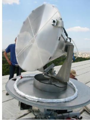
Figure 8: The heliostat being installed at the site of the pilot installation in Athens
