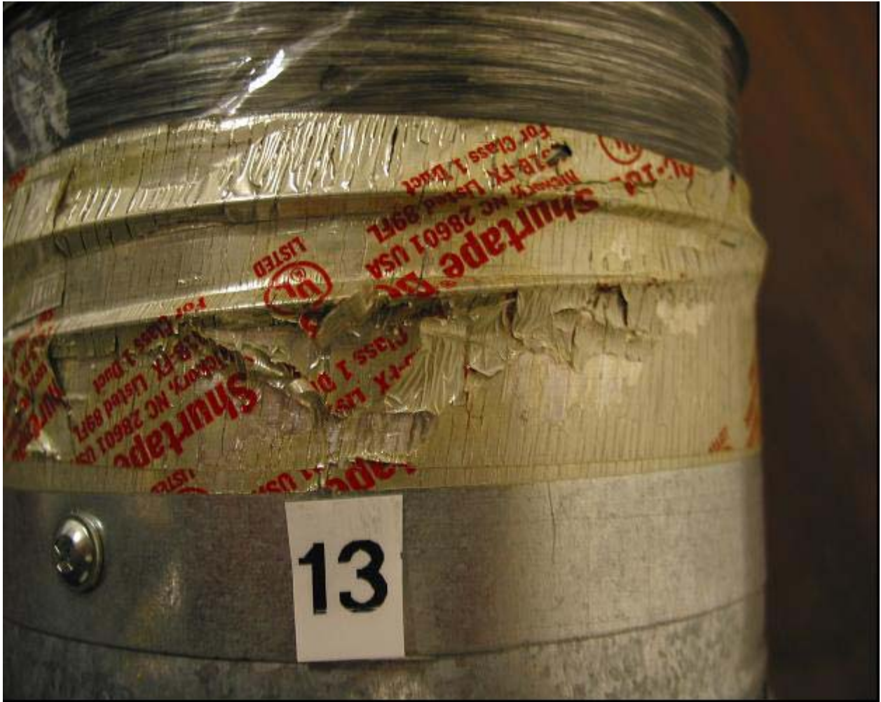
Figure A16. Sample 13. This sample is cracking and peeling.
