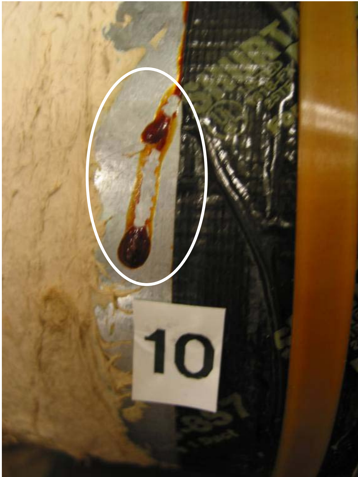
Figure A12. Sample 10. The adhesive has oozed out onto the surface of the duct.
