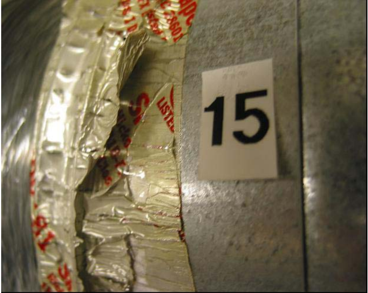
Figure A18. Sample 15. Like samples 13 and 14, this sample is also peeling and cracking. This figure shows how the metallized layer is splitting from the adhesive layer.
