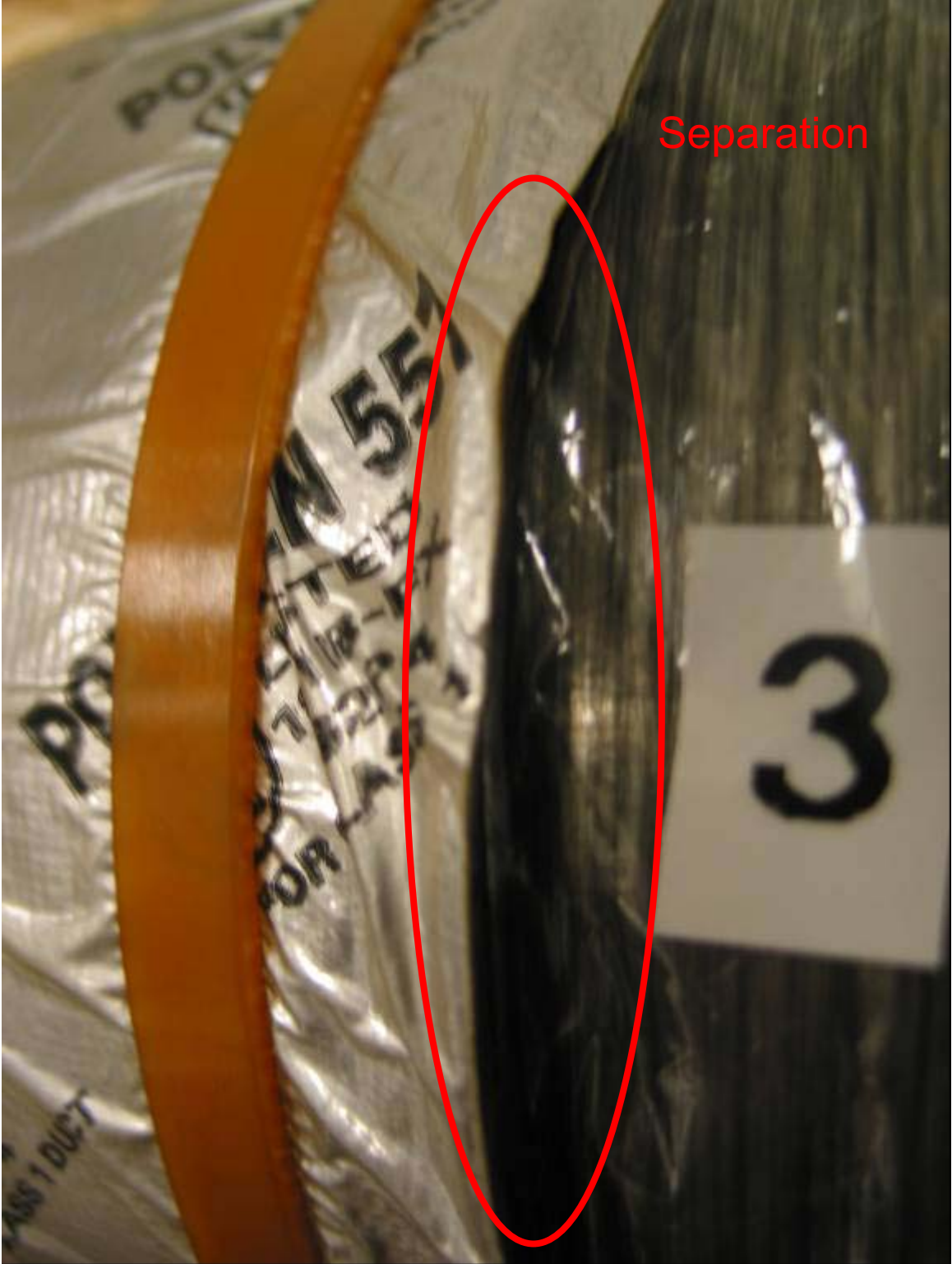
Figure A4. Sample 3. Tape has separated from the flex duct core at the tape edges
