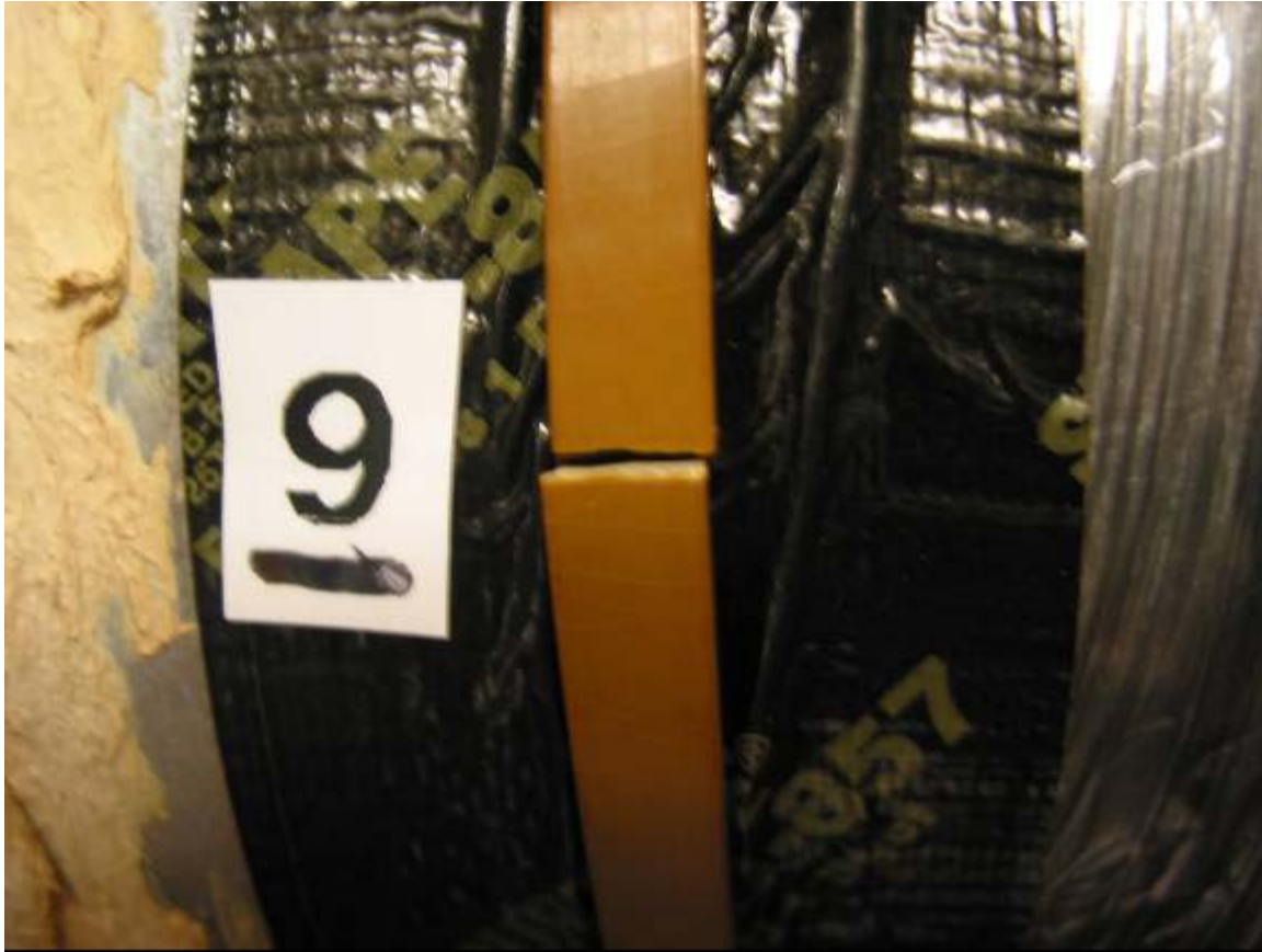
Figure A10. Sample 9. The clamp shows its brittle failure. Note that these clamp sections are now held in place because they are stuck to the duct tape.
