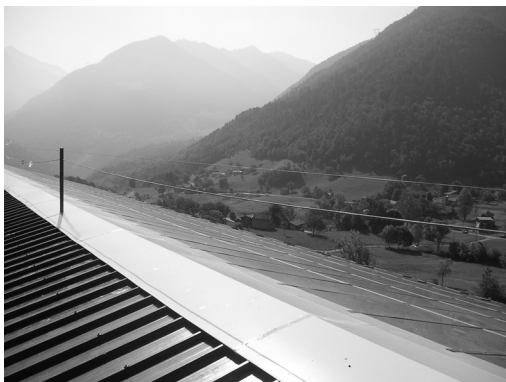
Figure 2: View of the solar integrated roof.
