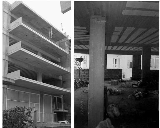
Figure 2: Views of the building of the second case study during retrofitting actions. Reconstruction of the building's envelope outside (left) and inside (right).
