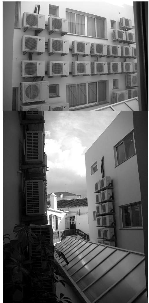
Figure 1: Two views of the air-conditioning system in a hotel central courtyard – the outdoor units of individual split systems for each room.
