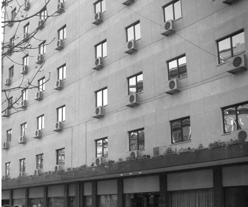
Figure 2: View of the main façade of a hotel using individual AC split units for each room.
