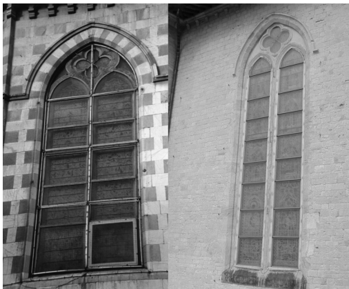
Figure 6: Old protective glazing system and new passive system installed in two different windows with the same orientation.
