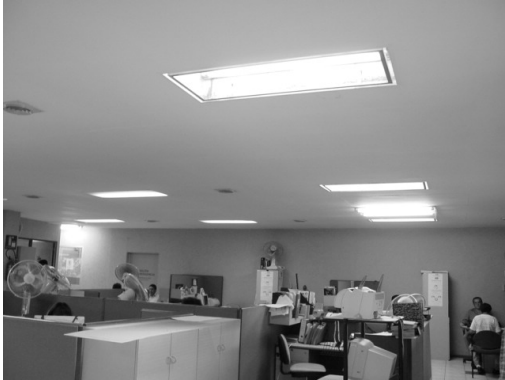
Figure 4: Internal view. Intensive use of lighting fixtures and electromechanical equipment during daytime working hours.
