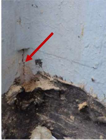
Figure 1: Breach in fluid-applied air barrier
