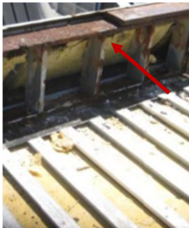
Figure 3: Corrosion on metal framing due to air leakage causing condensation
