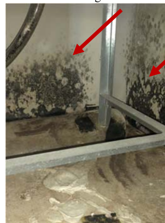
Figure 6: Mold growth on wall due to air and water leakage
