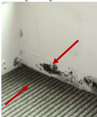
Figure 5: Mold growth on interior wall and damaged carpet due to air and water leakage
