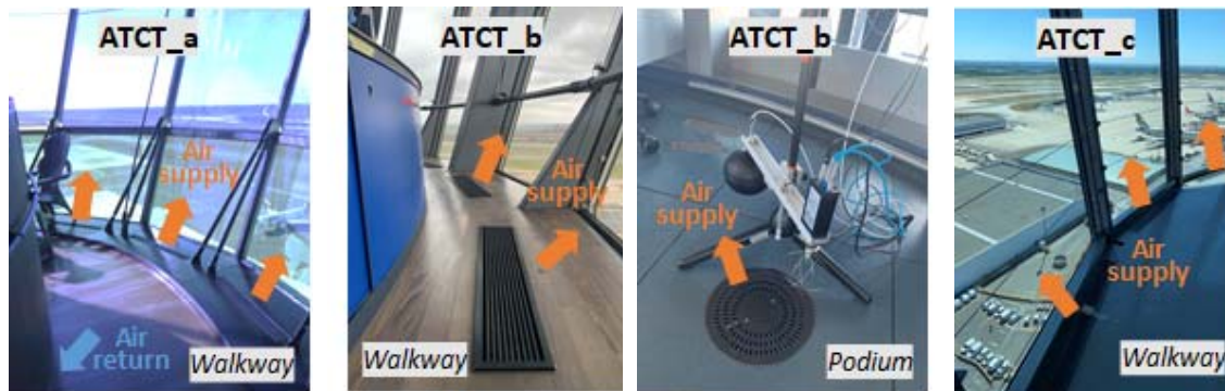
Figure 2. View of the supply air units in ATCT_a, ATCT_b and ATCT_c
