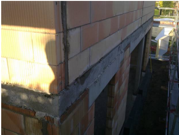
Figuur 10: The ends of the hollow core slabs have been filled with concrete
