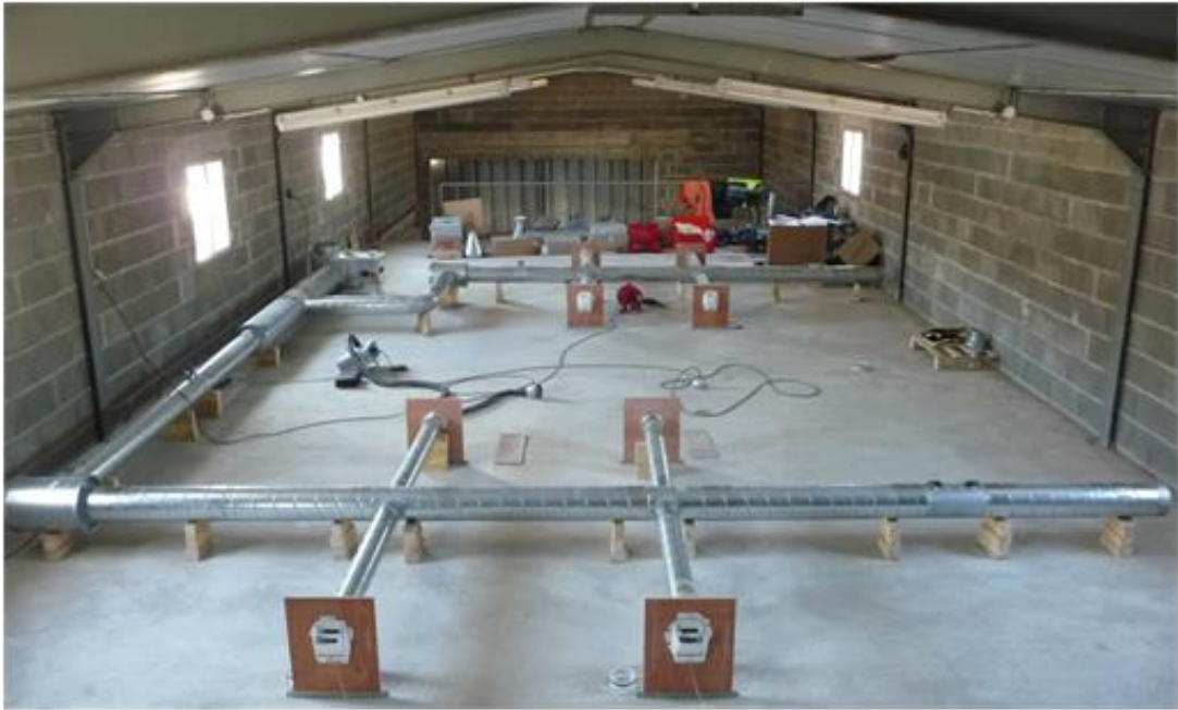
Figure 1: The ductwork studied
