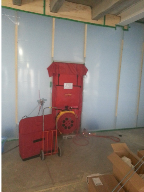
Figure 2. Temporary box filled with smoke for early stage testing and to identify leakage sources from outside of the building
