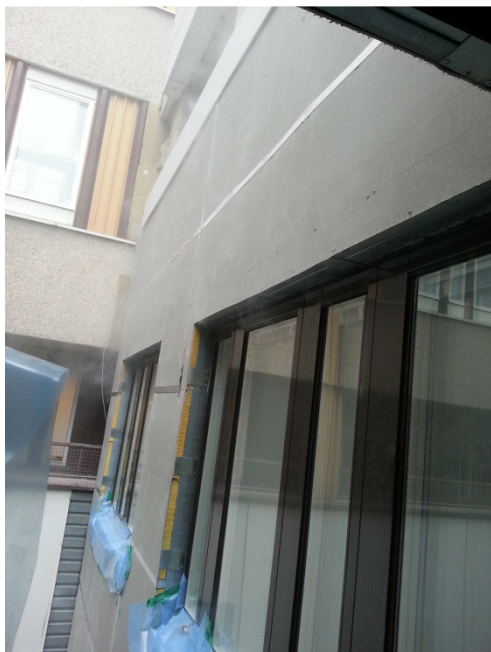
Figure 3. Smoke coming thru the outer wall and connection to existing parts of the hospital during pressurising test at +50 Pa.
