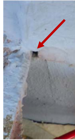
Figure 2: Breach in fluid-applied air barrier
