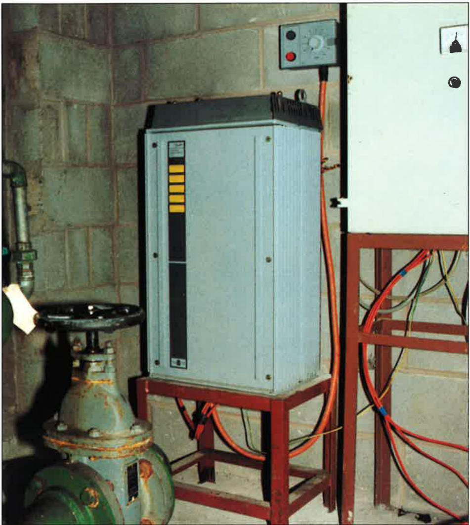
Borehole pump VSD with former throttling valve.
