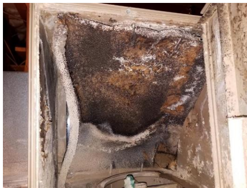
"Bypass humidifier" http://www.eiowainspections.com
