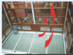
Figure 3(a) Bottom of a light-well: air rises vertically past heating fins and then through BMS-controlled louvers into library.
