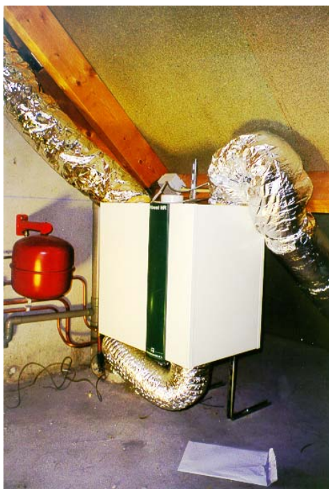
Figure 21 An example of a poor quality installation
