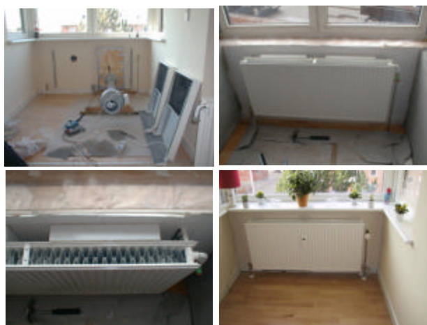
Figure 6.8 Illustration of a construction of the inlet from the solar wall, installed on a balcony.
