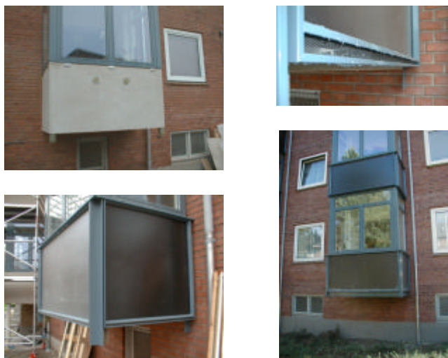
Figure 6.7 Illustration of a construction of a solar wall on a balcony seen from the outside. Housing company Østerbro, EU project FLEXREN.
