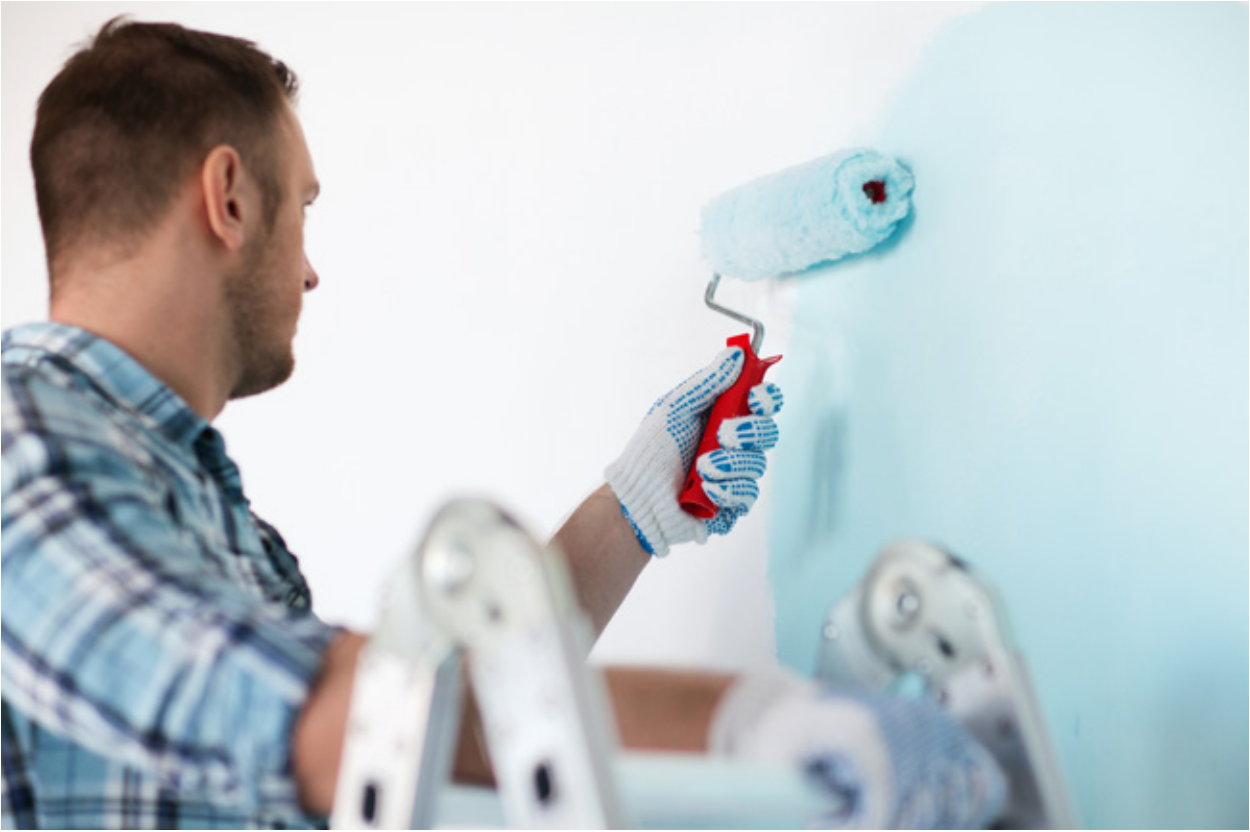
Figure 3: Paint can be a source of different pollutants
