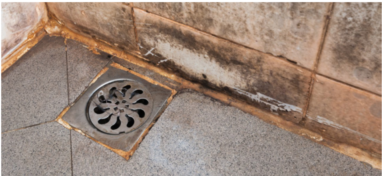
Figure 2: Mould in a bathroom
