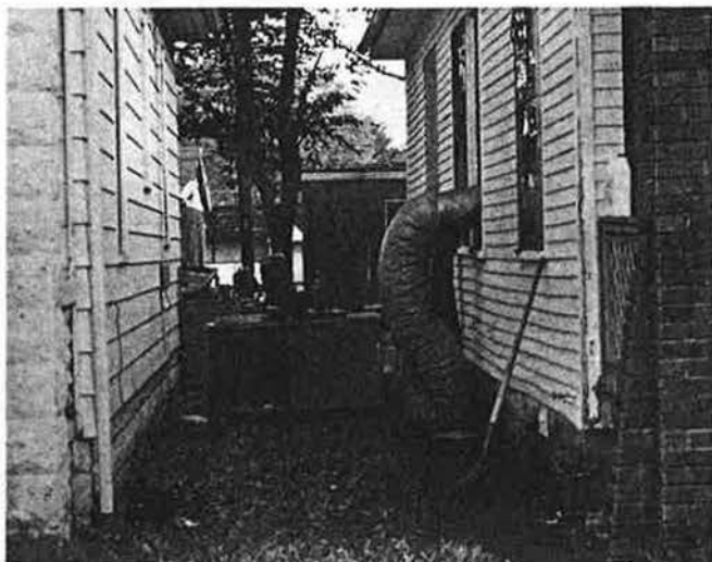
We're not sure what manual the installer of this creative air conditioning system was working with, but we don't recommend it!
