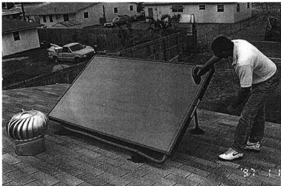
An installer measures the angle of a solar hot water collector atop this Miami, Florida roof. The sunny climate of the area makes solar water heating an attractive and relatively cost-effective retrofit.
