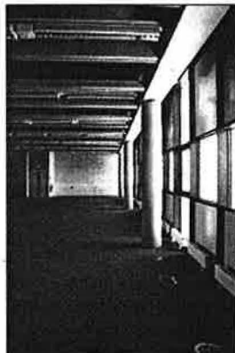
ABOVE: Ventilation air is distributed in ductwork under corridor floors, and into a supply plenum formed by the raised floor. Return is from a ceiling terminal housed in a quirky black-painted spigot, which passes air into return air ductwork in the raised floor above. High-frequency fluorescent lamps in modified Zumtobel luminaires are suspended in the exposed soffit grid.
