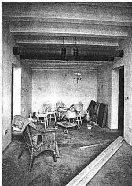
Inside the houses. The mechanical ventilation uses clay pipes slung from the high-mass structure. The pipes extend for the full length of the housing development, with spigots supplying the front rooms, and extract from kitchens and bathrooms.
