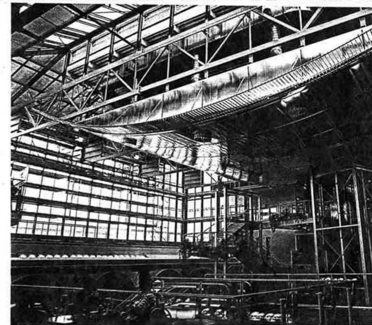
5 th View into the atrium with the central air treatment unit on a supporting structure under the dome. The supply air flows down through air outlets in order to avoid spreading smells.
