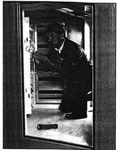
Technician adjusts air dampers in an outdoor AHU.
