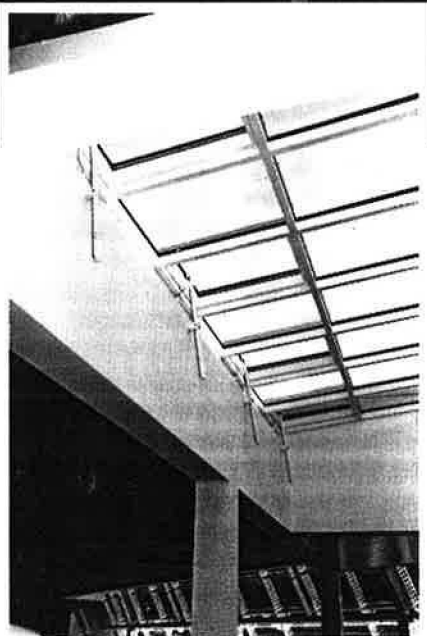
Rooflights incorporating actuator-operated windows open and close as part of the ventilation strategy.
