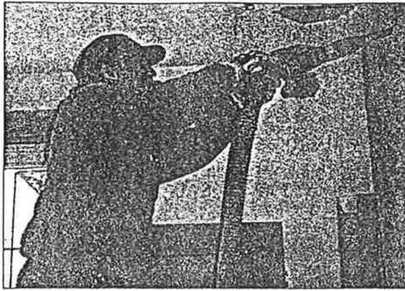
Added insulation is a commonly recommended energy efficiency improvement.
