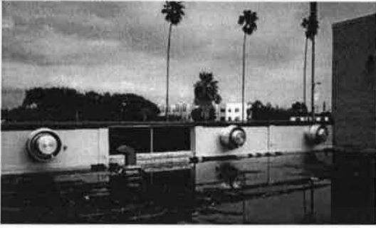
ASHRAE Info: Photo #3 Side wall exhaust fans on apparatus room exterior wall, located above living quarters roof.
