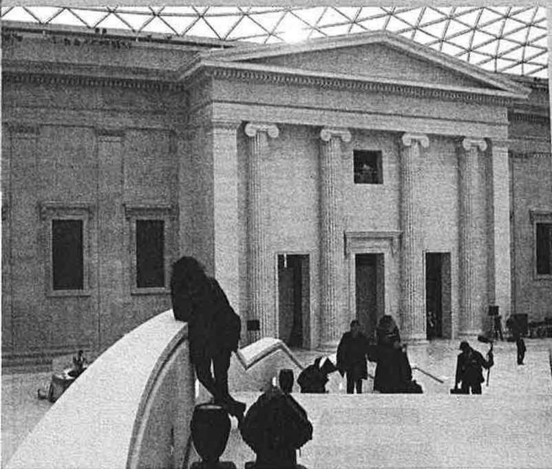
ABOVE: The Great Court's south portico, demolished at the turn of the last century, has been rebuilt in French oolitic limestone rather than the Portland stone of the original walls. The reading room has been clad in Spanish limestone.
