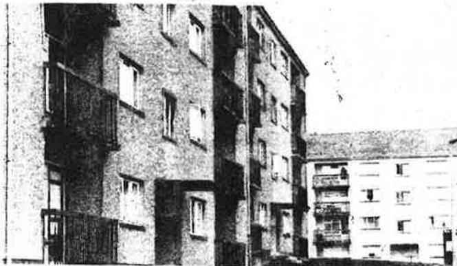
Flats at Stirling, Scotland, site of BRE studies of remedies for condensation.
