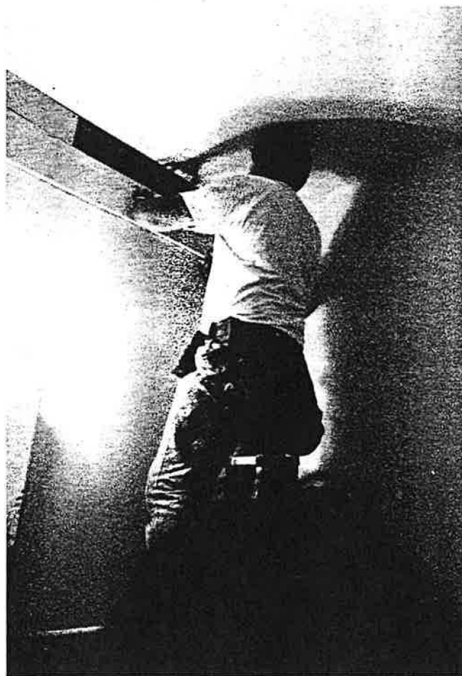
This wall is being repaired because it was tested with a blower door and an infrared camera and found to have no top plate.
