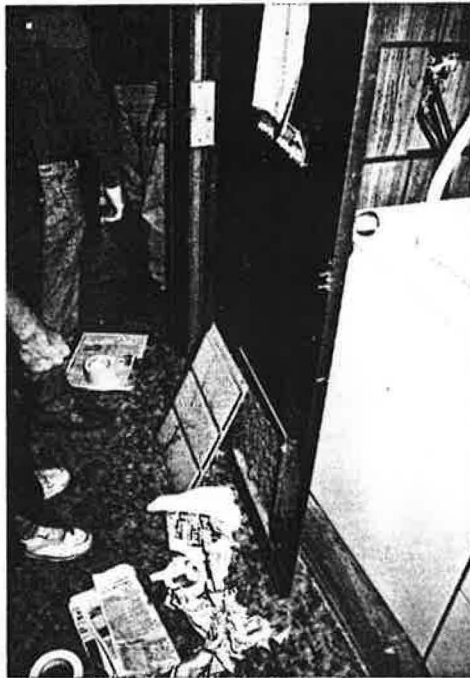
Accumulated dirt in furnace room return air grilles can be one cause of poor air circulation.
