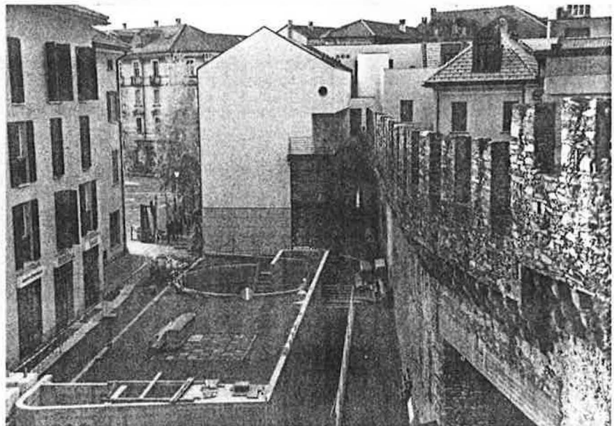
On the right the building complex during the retrofitting operation. Part of it is inside the old walls that surround the town of Bellinzona.
