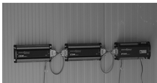
Figure 3: The datalogger and the channel expansion modules inside a box.
