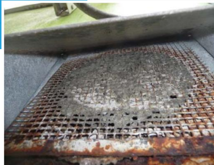
Dirty outdoor air intake.
