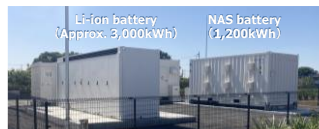
Additional batteries installed for the effective use of renewable energy after the construction completion
